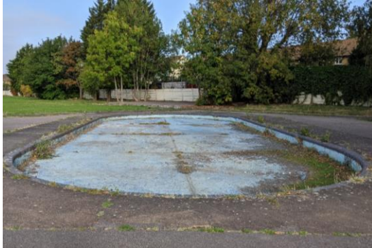
Plumstead Gdns– Derelict paddling pool remove and re –landscape
