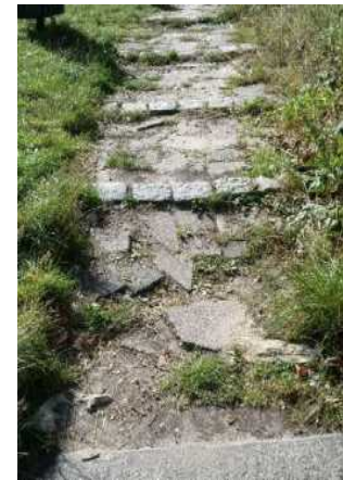
Shrewsbury Park – Broken dangerous path repair
